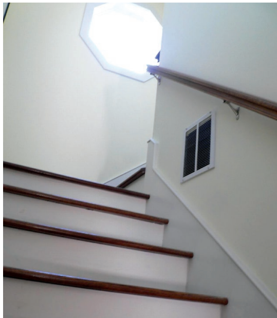
A grille at the peak of Dugan's top-story living room draws air into the dehumidifier (top) whenever the dehumidistat activates it. An always-on air-mixing fan pushes the dried air down to a basement stairwell register (above).
