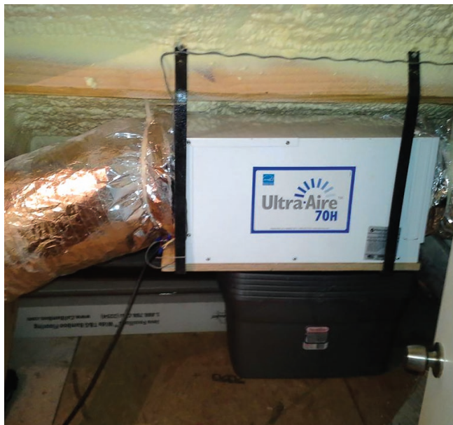
North Carolina builder Tom Dugan installed this Ultra-Aire 70H in his own home. The unit is rated at 70 pints per day and 5 pints per kWh. Dugan tied the dehumidifier into his already installed fan-powered air-mixing duct, which sends air from the home’s highest point down to the ground level.
