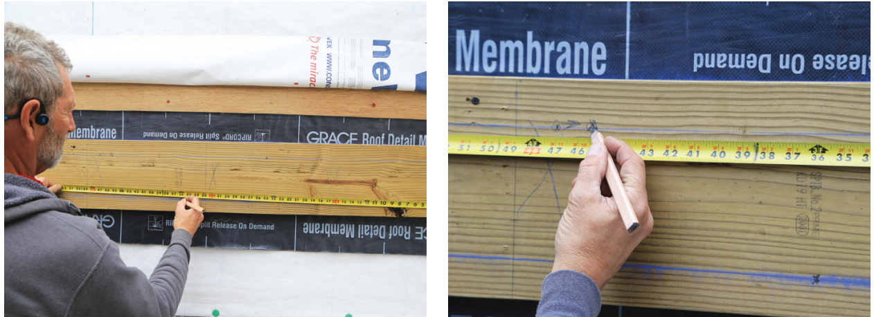
Figure 3. Fasteners are laid out on the ledger in two rows, starting approximately 3 inches in from one end, with the on-center spacing from the code table staggered in a “W” pattern between the two rows. Since bolt and lag heads can’t be countersunk into the ledger, the fastener can be moved left or right up to 3 inches to avoid conflicting with joist location or the hanger flange, provided the rest of the fasteners remain on the same layout.
