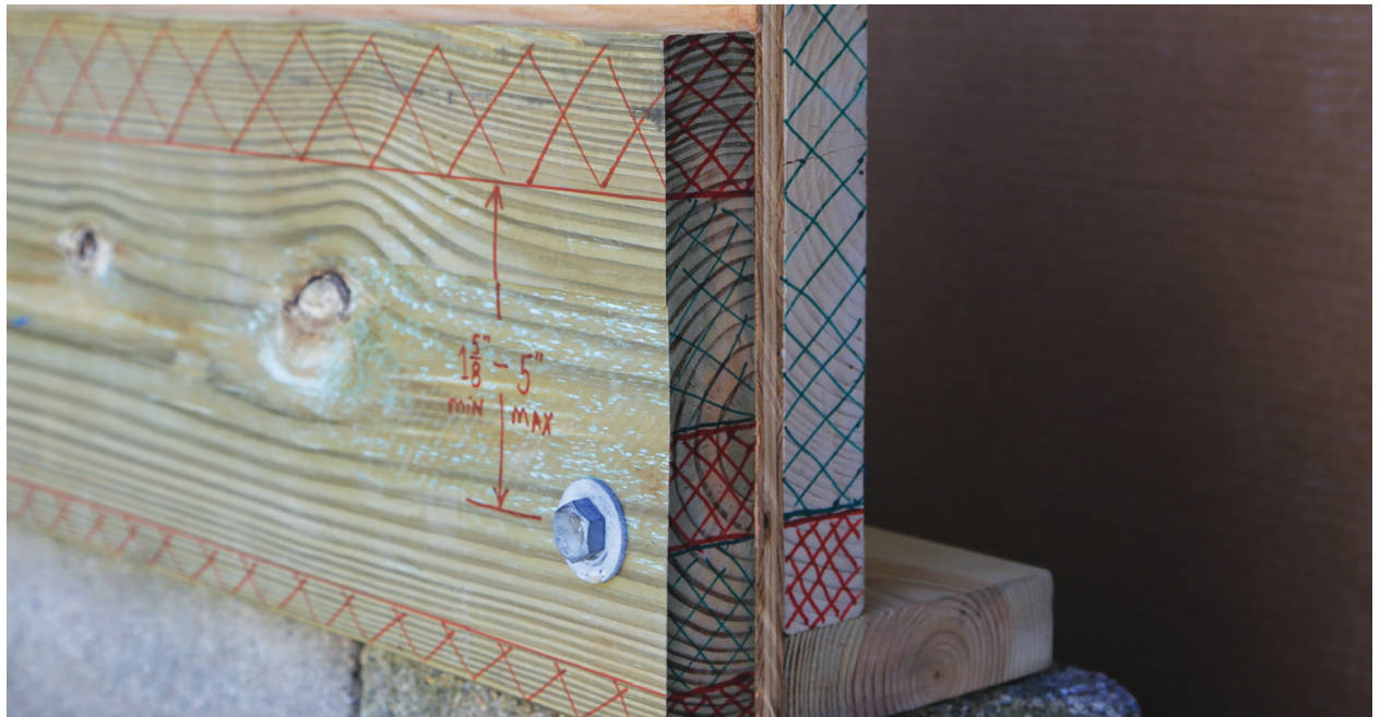
Figure 5. Applying the code figures when fastening a ledger can be confusing. The fastener locations through the ledger and through the rim joist differ, so you have to match the zones to ensure that the wood doesn't split and that you provide enough support for the deck.
