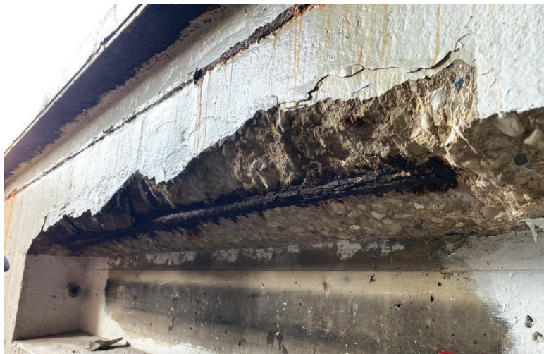
Rebar encased in concrete can still corrode, but the process is typically very slow. The surface corrosion shown here doesn't affect the steel's structural integrity and can be cleaned off prior to repriming and concrete repair work.
