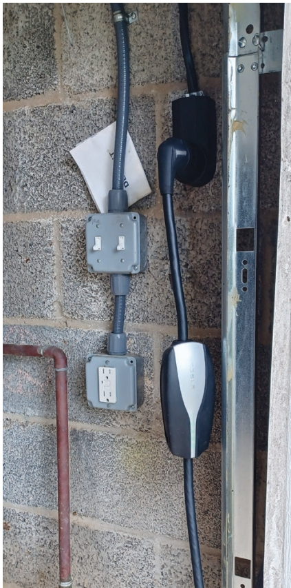
A NEMA 14-50 receptacle wired with a 6-gauge cable running back to a 50-amp breaker in the service panel will work for most mobile connectors.
