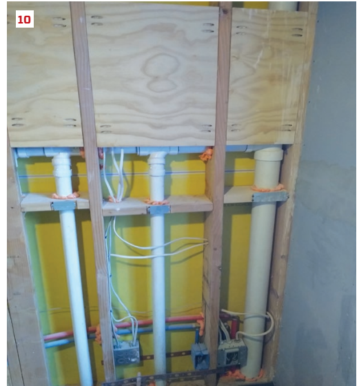
Air-sealing is not relegated to one phase of construction. Throughout the entire build, we continually seal anywhere air can penetrate or convect, as seen in this interior plumbing wall after the shell was sealed (10). Reducing air movement in walls is also important for improving fire safety, deadening sound (sound travels through air), and reducing unwanted moisture movement. In this case, these walls will be tiled on both sides.
