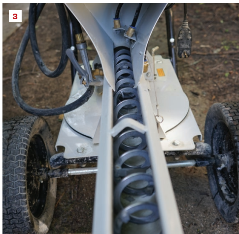
The mixing is done by an auger running the length of the narrow, horizontal chute (3).
