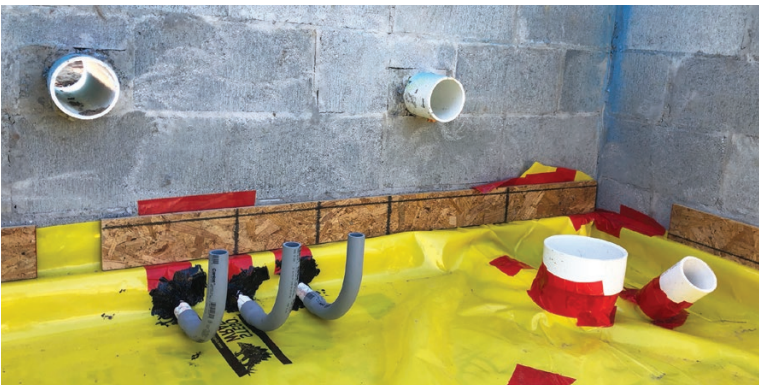
Stego Mastic (black goop around penetrations) and Stego Tape (red) prove effective for sealing Stego Wrap—a thick, polyolefin plastic specifically designed as a subslab vapor retarder.
