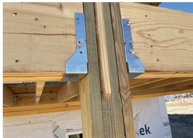
Figure 6. When connecting beams to continuous posts, choose metal hardware sized to fit the posts as well as for the loads. Here, the connectors have inward-turning flanges.
