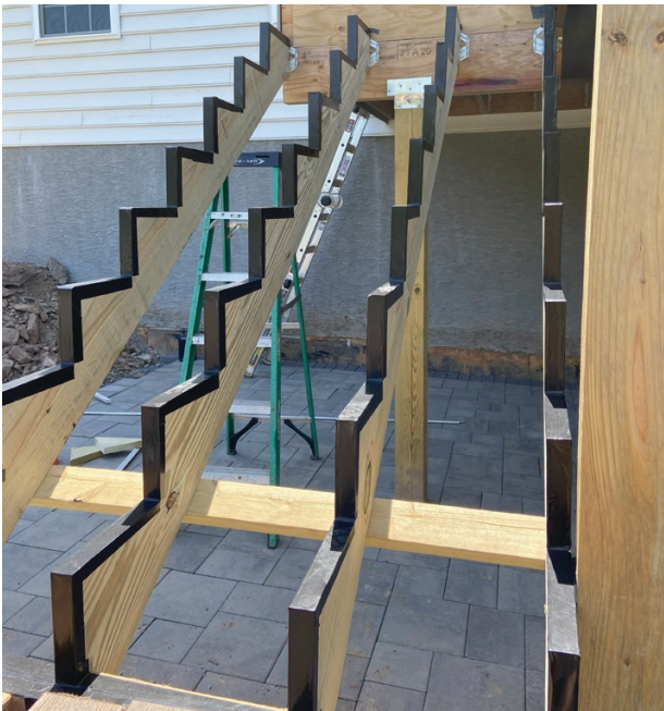
Cutting a stringer creates “end grain” at each stair tread and riser. End grain absorbs water up to 100 times faster than the sides of the lumber do. As such, cut edges of the 2x12 preservative-treated southern pine stringers are flashed.
