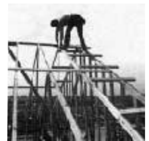
Installing outriggers and sway braces. With the four-truss sway brace in place, the last of the outriggers is nailed up. Once bracing is completed and a straight line snapped on the rafter tails, the roof will be ready for sheathing.
