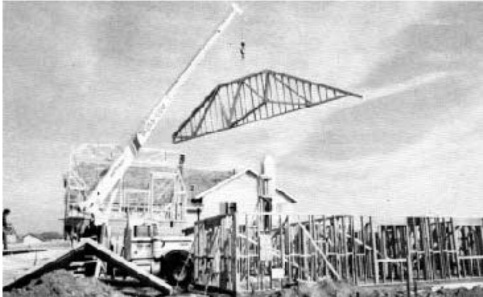
When trusses are set with a crane, both speed and safety depend on crew and crane operator being in sync.
