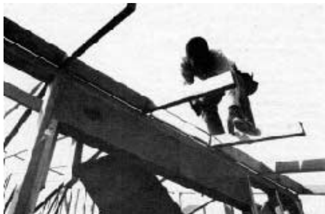
Nailing in frieze blocks. Vent screens and frieze blocks not only finish off the space between the truss tails in this open-soffit design; they also maintain the 2-foot on-center spacing. The plywood "special" hanging from the header will be used to keep ceiling insulation from blocking the vent.
