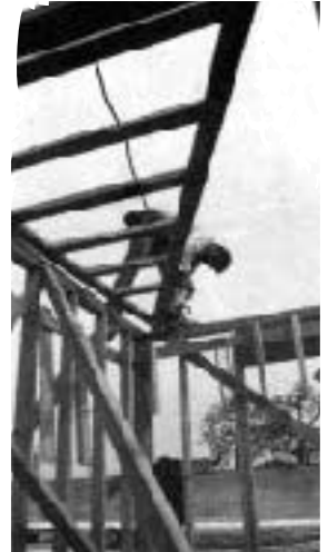
Prepping the gable end. Working on the plates, this carpenter has preset toenails on the bottom chord of the gable truss and is cutting notches for the outriggers. Note the frieze blocks, vent screen, and outriggers hanging from the 1x4 ledger, which keeps these "accessories" in reach.
