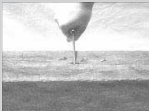
Pick test. A short splinter pried from decayed wood (left) typically breaks quietly over the tool with both ends still anchored. When pried from sound wood (bottom), the splinter cracks sharply, is longer, and remains attached at one end only.
