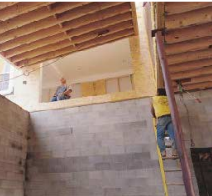
Figure 4. After the modular boxes are craned onto the foundation (top), the set crew bolts the floor systems together and supports the “marriage wall” — the common wall between boxes — using adjustable steel columns (above).
