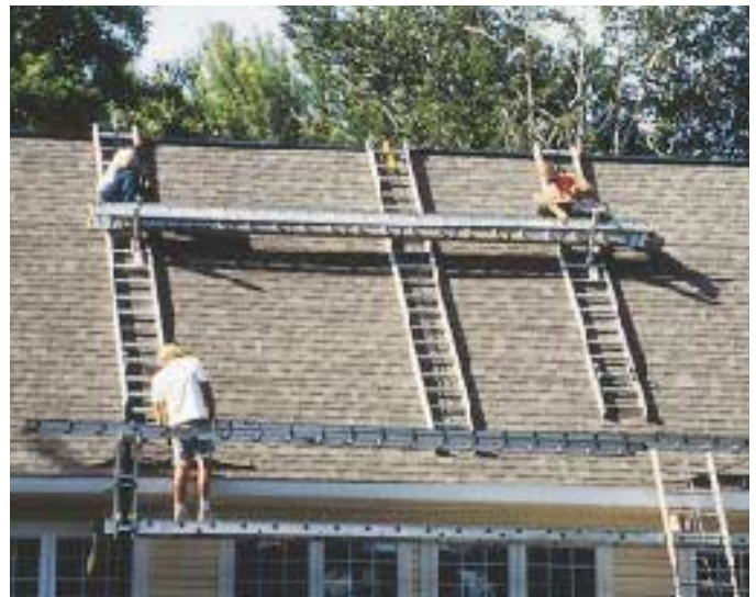
Figure 5. The roof, which is hinged and folded back on itself for shipping, is craned into place (top) and supported, either temporarily with posts or permanently with a structural ridge or pre-assembled kneewall. In a custom design, prebuilt dormers or second-story walls may also need to be placed by crane (middle). The last step is to weave several courses of roofing into the unfinished areas (above).
