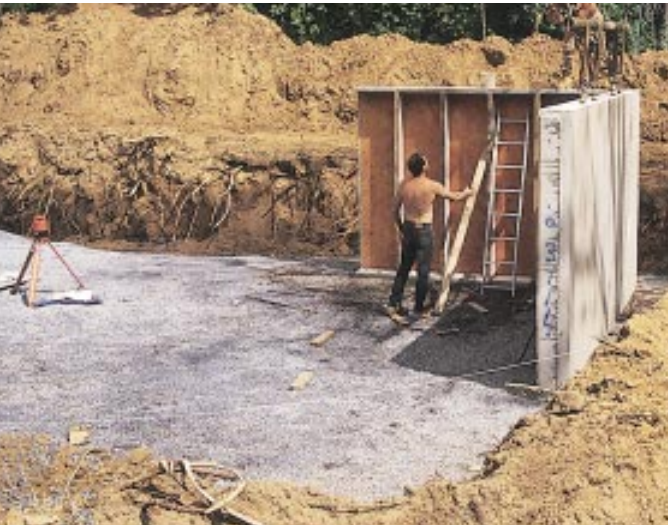
Figure 3. To take delivery, the site must provide clear passage for a tractor trailer (top). The foundation crew handles the excavation and uses a crane to place precast concrete walls (middle and above).
