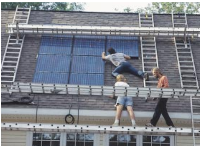
Figure 6. Once the modular sections are set and buttoned up, the author's crew completes special features, such as radiant heating (top) and photovoltaic panels (above), on site.
