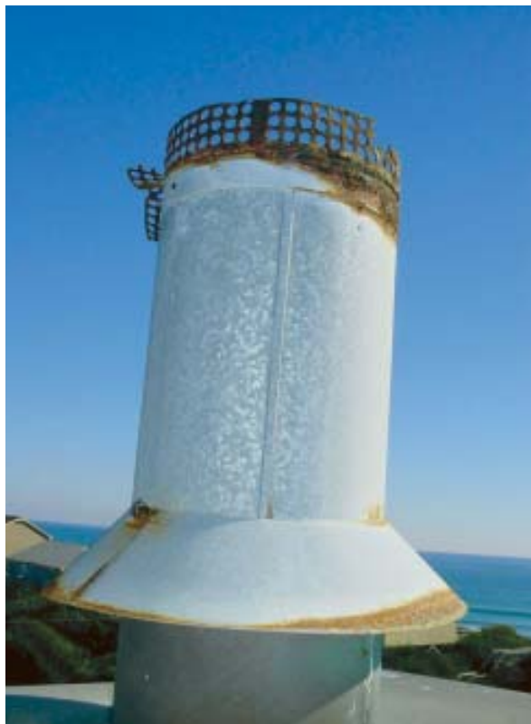
Figure 2. Most failed or failing prefabs are discovered in the course of a routine chimney cleaning, not because the homeowner realizes something is wrong. A missing termination cap (left) or leaking chase cover can quickly cause internal rust. This sort of damage is often evident around the damper at the top of the fire-box (below) or behind the louvers of a circulating fireplace (bottom).
