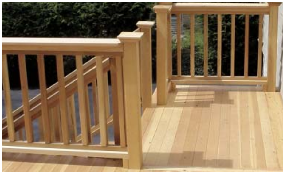
FIGURE 1. On outdoor decks, Peter Kroll of North Falmouth, Mass., prefers vertical-grain fir for its tight grain and the ready availability of mixed lengths. He doesn't oil the wood; instead, he allows it to weather naturally. This reduces the maintenance for clients, as any outdoor finish would have to be reapplied every couple of years in a coastal environment.
