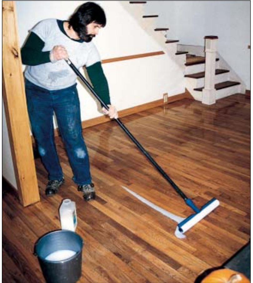
Waterborne finishes have a good track record of performance and, if properly applied, will outperform oil-modified urethanes. However, the learning curve for installing them correctly is steep.
