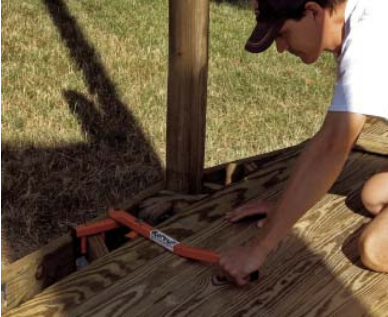
Figure 8. Crooked decking is made straight with one hand doing the pulling and the wedge-action of the BoWrench tool exerting an incredibly strong force.
