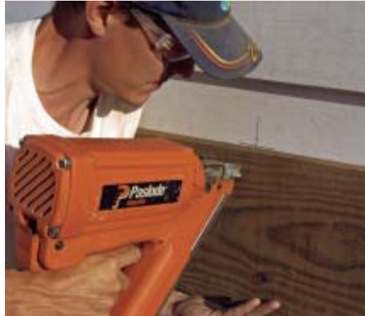
Figure 3. Here the author is installing the ledger board to the house, using a centerline marked on the board and aligned to match one that's marked on the house. A power nailer leaves one hand free to support the workpiece.
