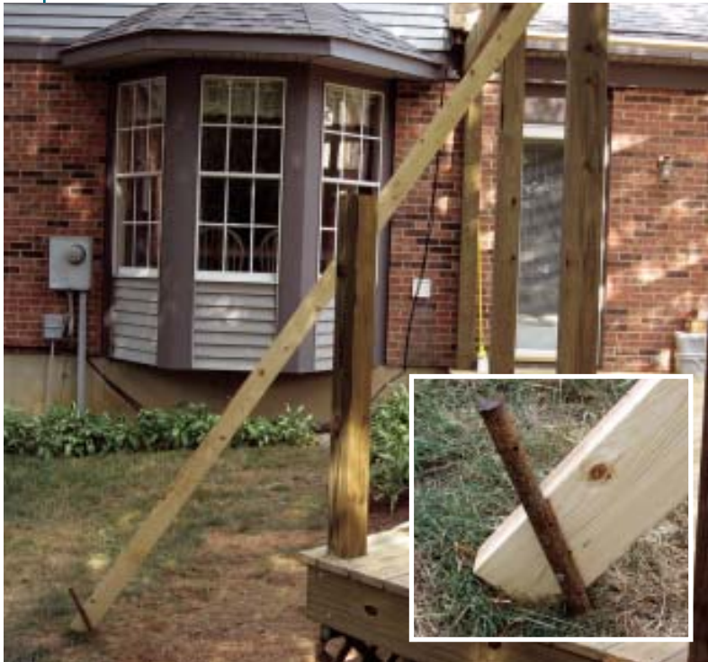
Figure 4. Posts taller than approximately 6 feet are braced with at least two 2x4s that are screwed or nailed to the posts on one end and tied to steel stakes driven into the ground on the other end.
