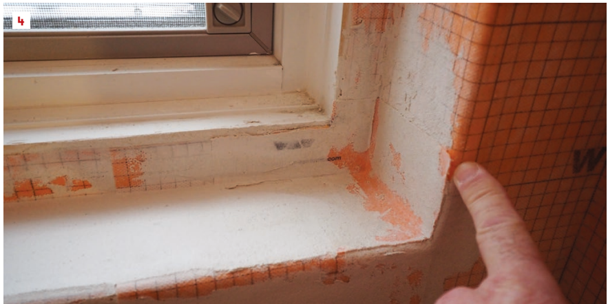
At an existing window in a new shower, the author's company installs Kerdi membrane, lapping it onto the window (2). This application is inherently risky, requiring near-perfect workmanship. The author identifies two instances (3, 4) where the membrane is not sealed and will need extra attention from the crew.
